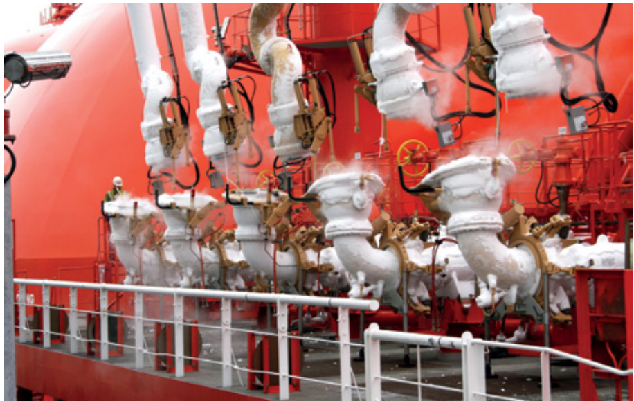
The Emergency Shutdown Systems (ESD) Working Group is focused on the revision of SIGTTO's previous guidance on the topic, issued in 2009
